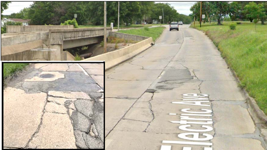
Electric where canal terminates. Inset showing extent of road damage typical of the entire street.
