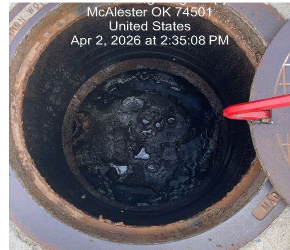
Grease Trap Outdoors (FULL)
