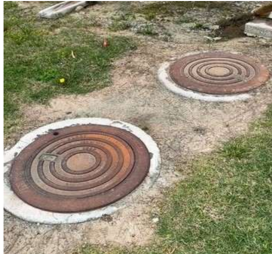
Grease Trap Outdoors
