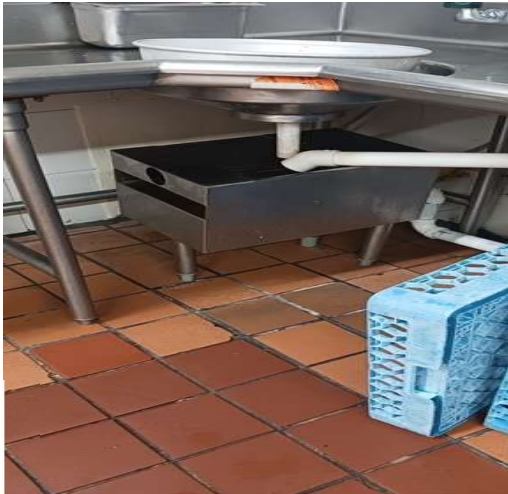
Grease Trap Indoors
